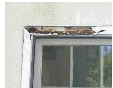
Wood rot to brick mold below kickout
