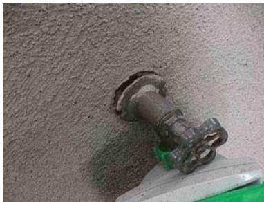
Hose bibb needs to be caulked
