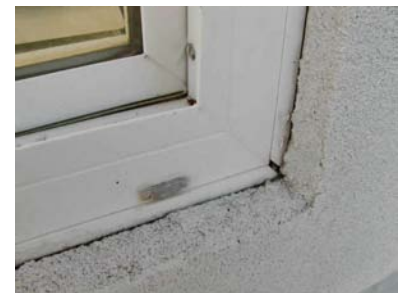
F-6: Large cracks at window
