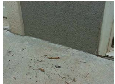
System in contact with concrete. No termite band.
