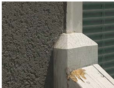
Paint peeling. Seal joint at house.
