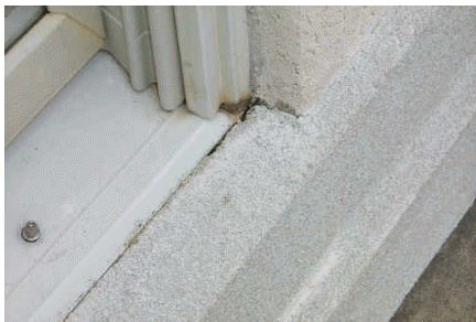
E-7: Window needs to be caulked
