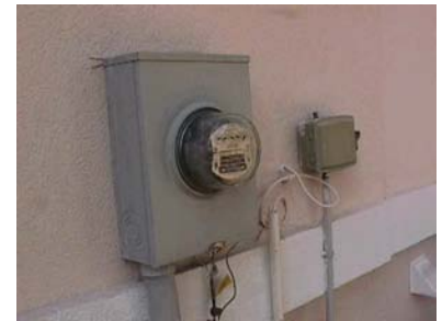
Utility breaches need caulk
