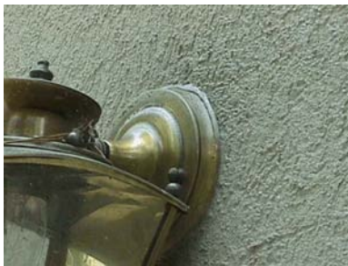
Light fixture needs caulk
