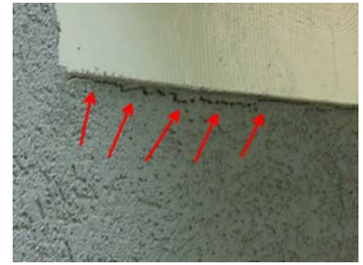
Exposed crack needs to be caulked
