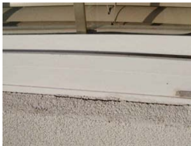
Typical exposed cracks at window
