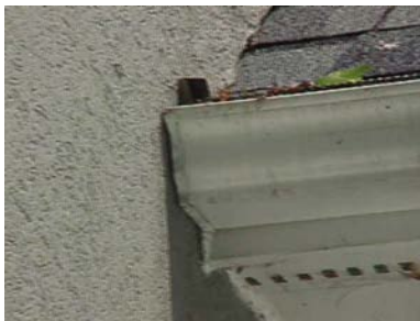
A-5: Kickout installed. Need to clean gutter.
