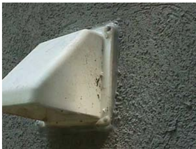
Vent needs to be caulked
