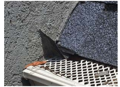
Kickout on right side of chimney
