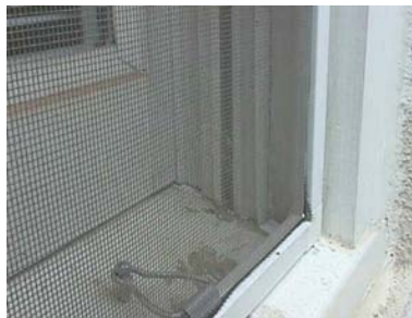
Miter joints not caulked
