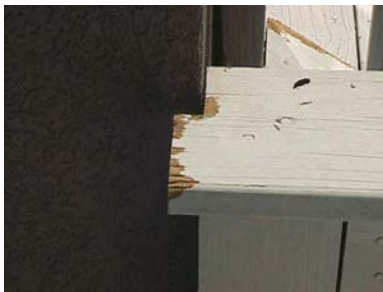
Paint peeling at porch
