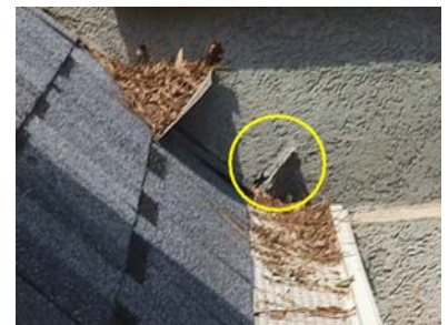
Kickout improperly installed. Clear leaves from area.
